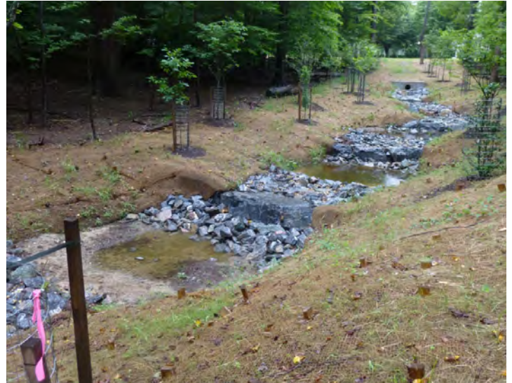
A drainage outfall at the Upper Watts Branch Forest Preserve has been redesigned from a straight continuous sloped channel, which caused erosion and flooding issues, to a ‘pool, riffle, run’ system where water can be slowed, filtered, and more easily absorbed as ground water.
