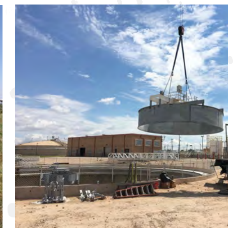
Lubbock water treatment plant Source: City of Lubbock
