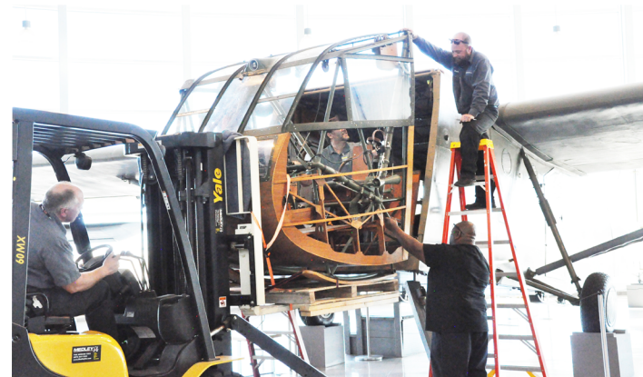
Temporary cockpit applied during work. This cockpit made by a different manufacturer made fitting a delicate operation.
